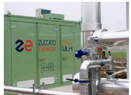
Borgoforte (Mantua, Italy) - Heat recovery from cooling jackets & exhausts of biogas-fueled gensets
