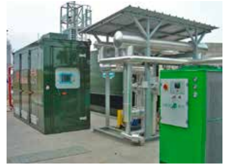
Portogruaro (Venice) - Heat recovery from cooling jackets & exhaust gases of biogas-fueled gensets
