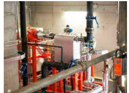
Mestre (Venice, Italy) - Heat recovery from biomass boiler and hot air turbines
