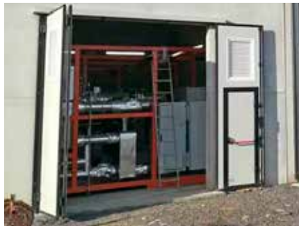
Città della Pieve (Perugia, Italy) - ORC power generation from biomass (pruning residues)
