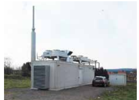
Benneckestein (Germany) - Heat recovery from cooling jackets & exhausts of biogas-fueled gensets
