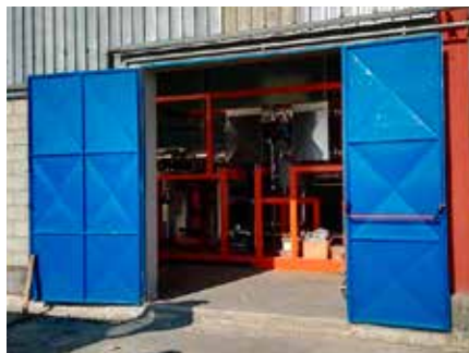
Castrovillari (Cosenza, Italy) - ORC Power generation from biomass (pruned tree branches)
