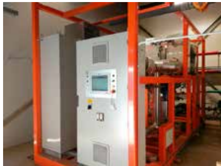
Rovato (Brescia, Italy) - ORC Power generation from biomass (end-of-life shipping pallets)
